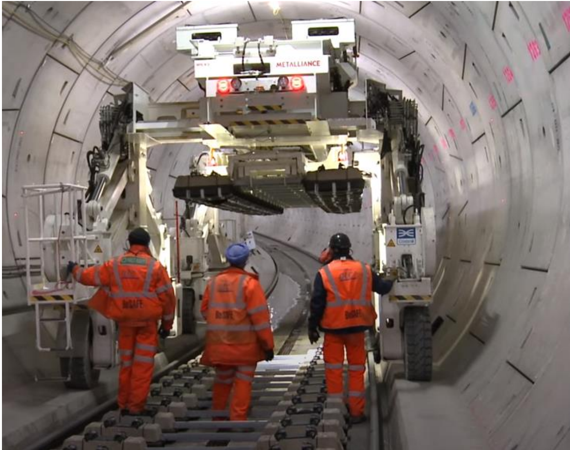
Diagram 2.14: Multi-Use Gantry Laying Sleepers for Crossrail. Note this is a Single-Track System, not Twin, as for the Proposed Project
