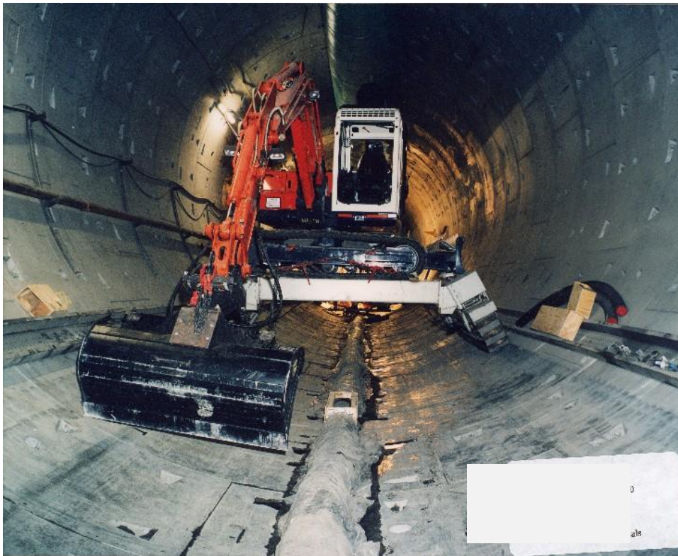
Diagram 2.12: Excavator in the Tunnel Which Places the Concrete in Front of the Paver
