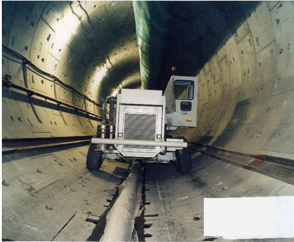
Diagram 2.10: Concrete Delivery Truck During Paving in the Channel Tunnel Rail link (CTRL)
